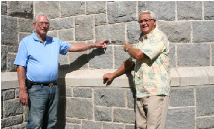
Al Vildibill, left, and Larry Fletcher point out bore drillings in the blocks in Grossmont High School's front wall.
